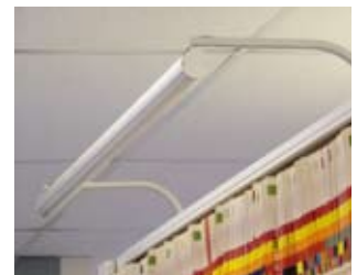
Overhead Aisle Lighting
