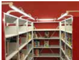
LED AISLE LIGHTING
