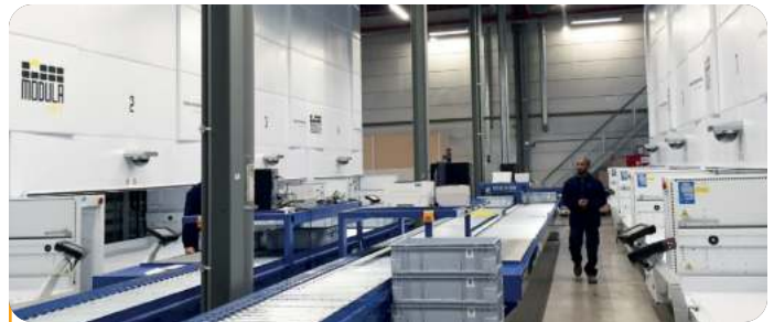
Integration with conveyors
